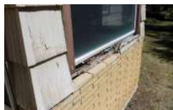
Ranger house in poor condition
