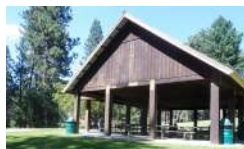
Pavilion in need of upgrades
