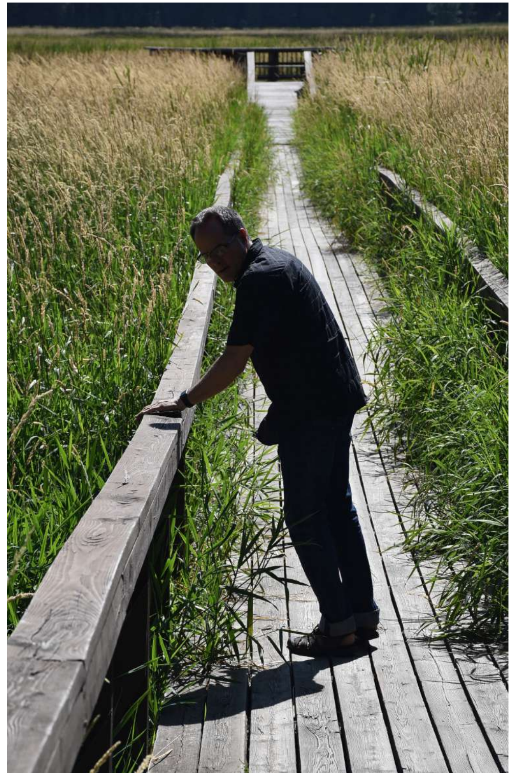
Existing boardwalk is in need of repair and upgrades for environmental education.
