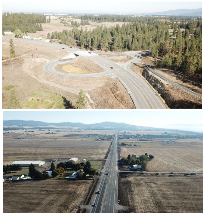
Figure 3: Completion of the grade separated intersection at Bigelow Gulch Road and Forker Road in 2019 (top) and reconstruction of a section of Bigelow Gulch Road between Argonne Road and Forker Road in 2019 (bottom)
