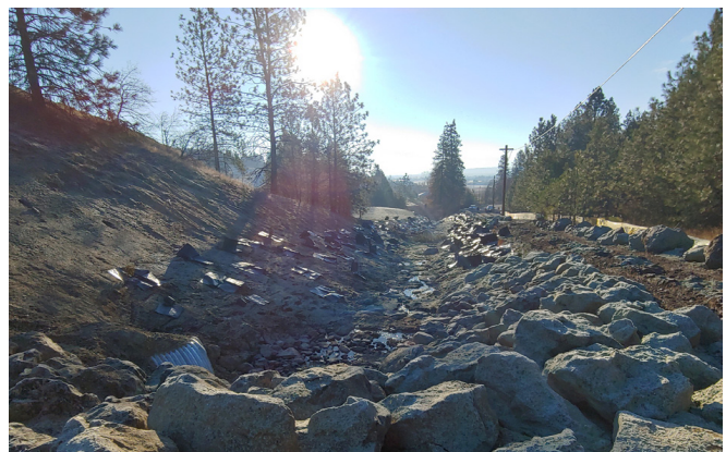
Figure 12: New culvert and stormwater runoff channel along an improved section of Bigelow Gulch Road
