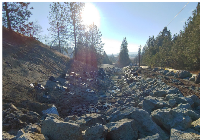
Figure 12: New culvert and stormwater runoff channel along an improved section of Bigelow Gulch Road
