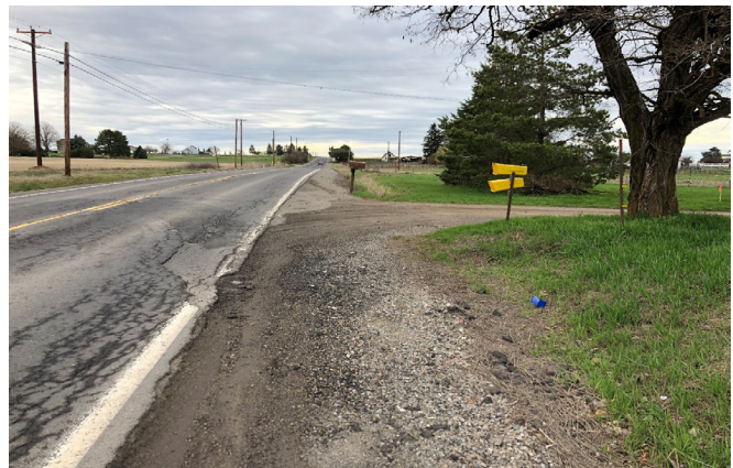
Figure 10: Pavement and shoulder conditions at the west end of Bigelow Gulch Road
