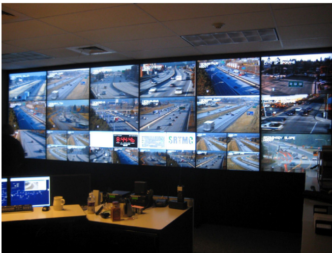
Figure 16: Spokane Regional Traffic Management Centre
