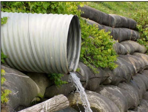
Figure 2. Storm Sewer MS4 outfall
