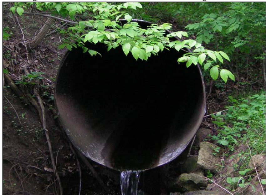
Figure 11. MS4 outfall location with illicit discharge
